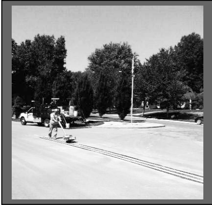
A city contractor applies double yellow lines to 69 th Street at Edgevale and Wornall in September.
